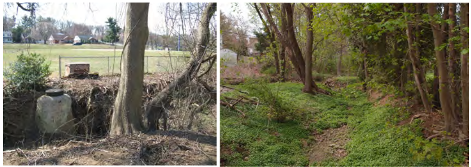
Left: Exposed manhole at Roychester park subject to erosion. Right: Historic channel at Grove Park.
