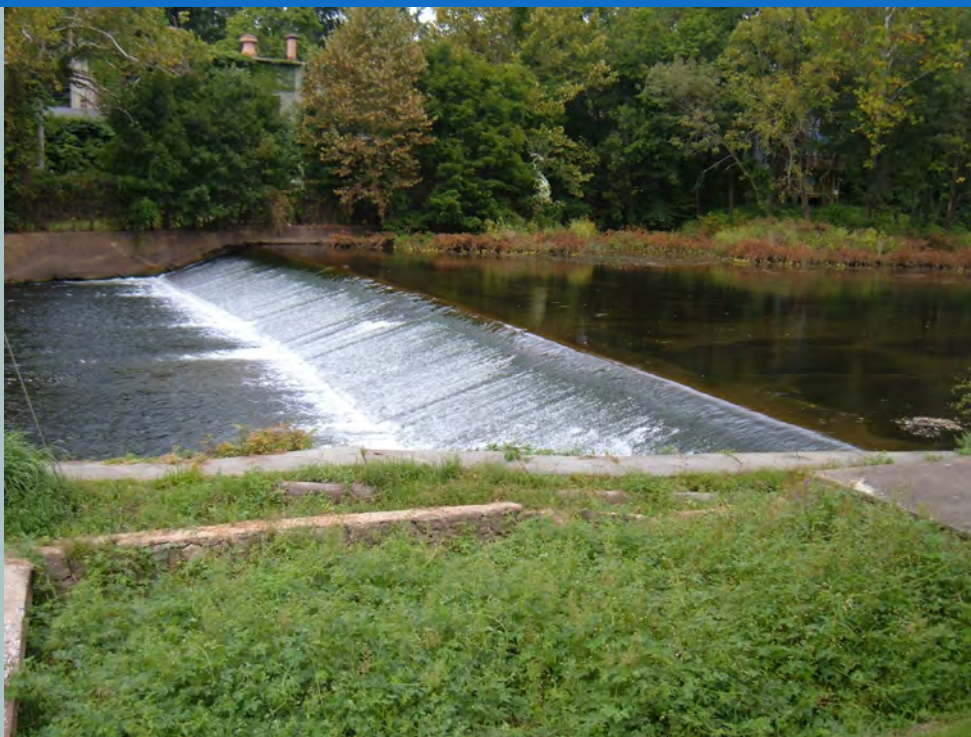
A view of the Bloomsbury Dam and the upstream impoundment area where natural river habitat conditions have been degraded due to the presence of the dam.
