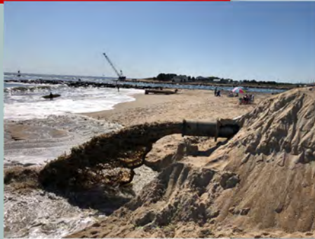
The state of Delaware operates the Indian River Inlet sand bypass plant in Sussex County, DE. Sand is pumped from the south side to the sand-starved north side. Federal construction funds
